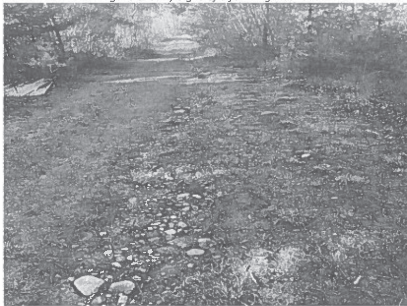
Figure 2: early signs of a forming washout
